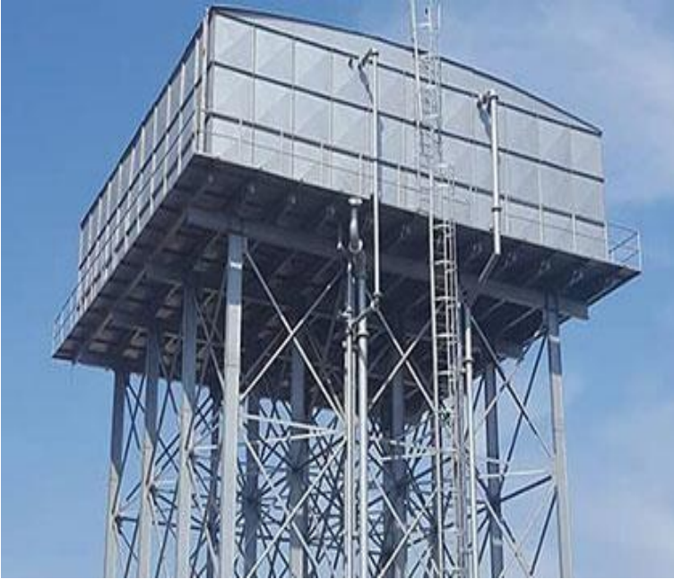
Figure 24: Elevated steel tanks
